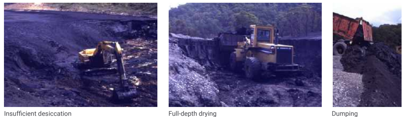
Figure 4. On-off coal tailings cells, employing solar and wind drying, harvesting and disposal with coarse reject
